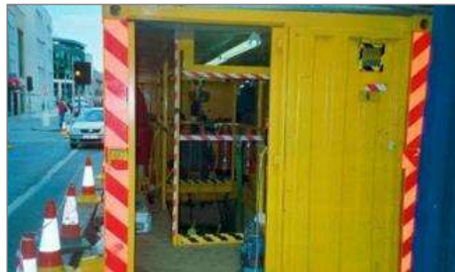
Figure 11 - HV cable jointing container
